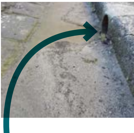
Sediment management: high risk of sediment washing into biofilter during construction in catchment
