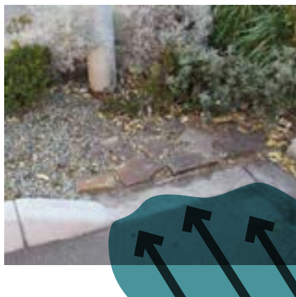
No step down into biofilter: flow cannot easily enter
