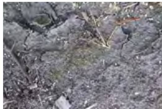
Clogging – build up of fine sediments, moss or plant litter on the surface reduces infiltration and treatment
