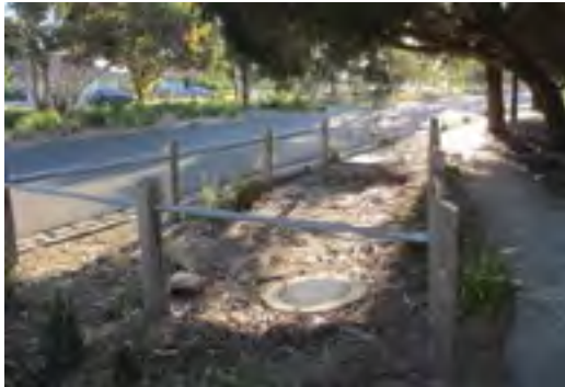
Widespread plant loss or die-back – can indicate too much or too little water, or poor filter function
