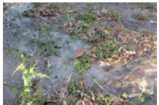
Weeds – unsightly and can reduce treatment capacity
