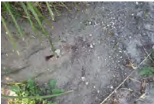
Sediment accumulation – build up of fine sediments reduces infiltration and treatment
