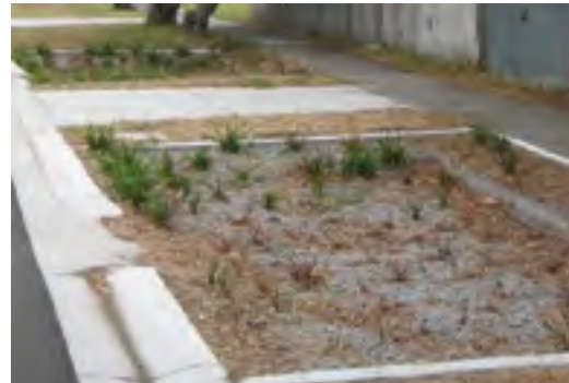
Plant die-back – severely reduces treatment efficiency and leaves media vulnerable to erosion
