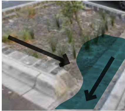
Surface of biofilter not flat, slope follows fall of road – poor distribution of flow
