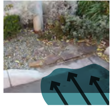
No step down into biofilter: flow cannot easily enter
