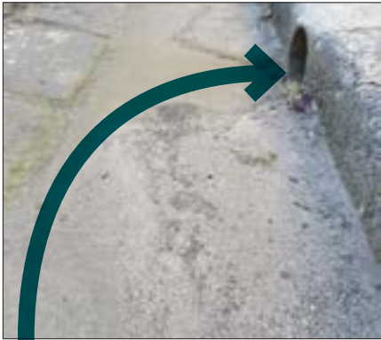
Sediment management – high risk of sediment washing into biofilter during construction activities
