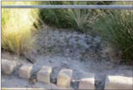
Plant die-back near inlet – may indicate high inflow velocities, sediment accumulation or poor species selection
