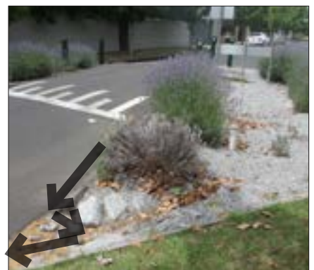
No drop down into biofilter and system overfilled with media and mulch. This prevents flow from both entering and ponding.
