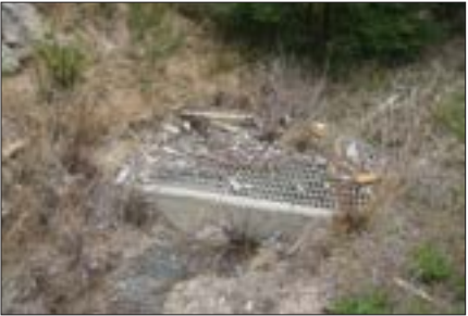
Blocked overflow grate – can lead to flooding and damage to the filter and vegetation
