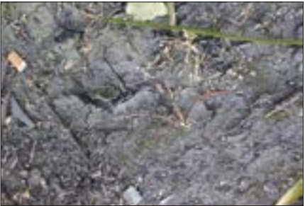
Clogging – build up of fine sediments, moss or plant litter on the surface reduces infiltration and treatment capacity
