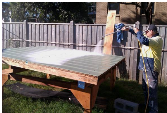
The extensive green roof treatment (upper) and the white elastomeric insulating ceramic coating (lower)
