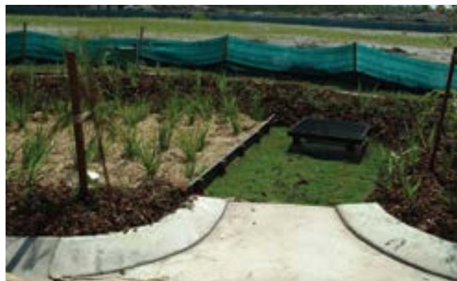
Figure 3. Concept illustration showing how Ag pipes installed for tree watering can result in short circuiting and reduced stormwater treatment.
