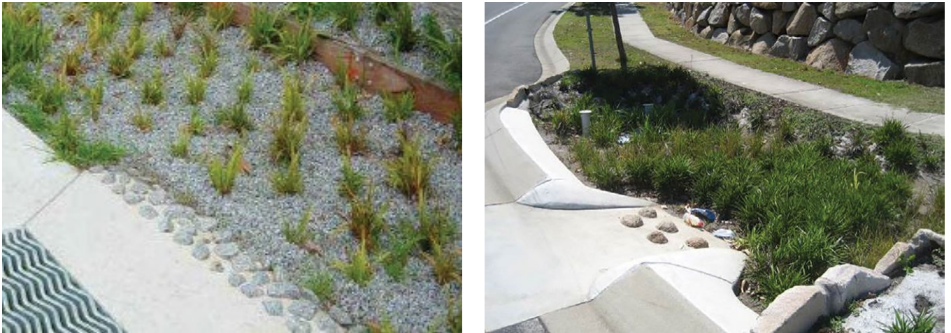
Figure 18. A rock apron (left) and dense vegetation (right) at the inlet to a biofilter can be used reduce flow velocities and prevent scour and erosion damage.
