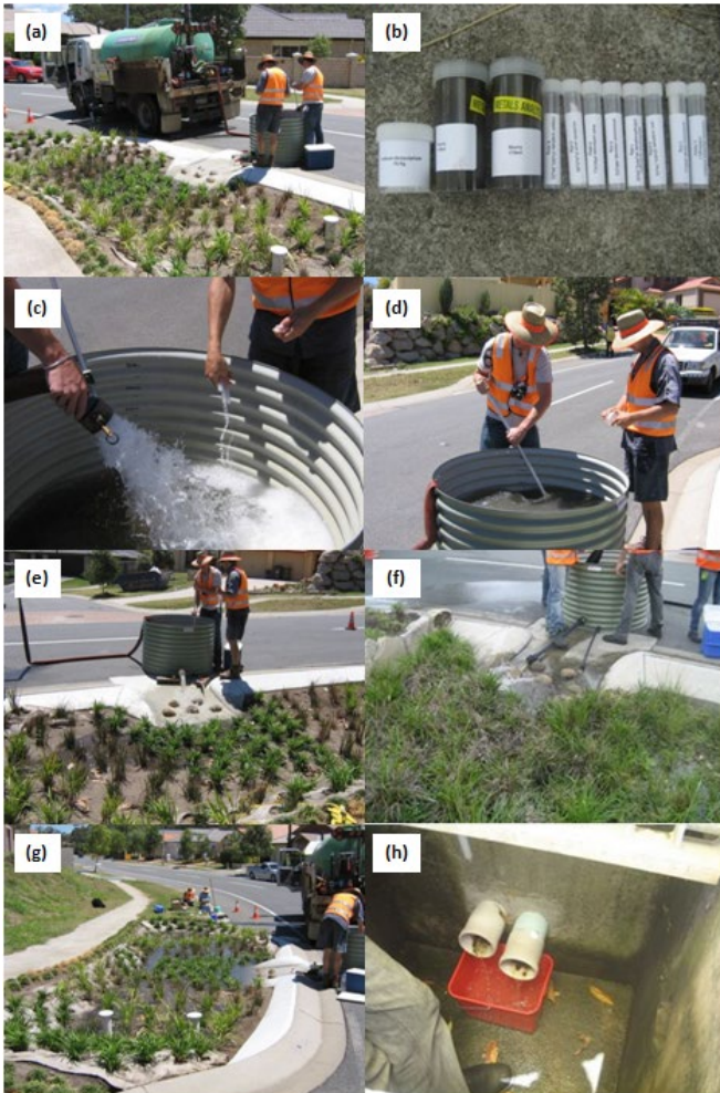
Figure 2. Conducting a rain event simulation at the Saturn Crescent biofiltration system.
