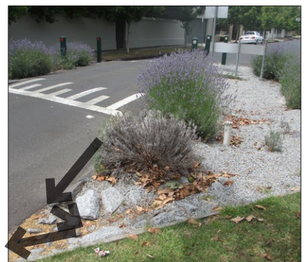
No drop down into biofilter and system overfilled with media and mulch. This prevents flow from both entering and ponding.
