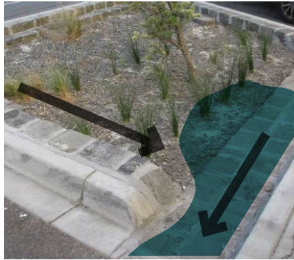
Surface of biofilter not flat, slope follows fall of road – poor distribution of flow
