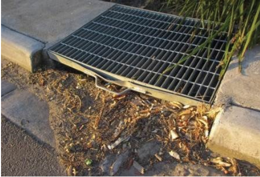
Blocked inlet – restricts flow entry, reducing proportion of flows receiving treatment
