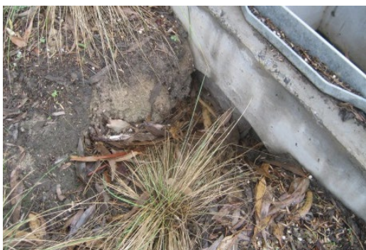
Holes, erosion and scour – compromise even flow distribution and treatment
