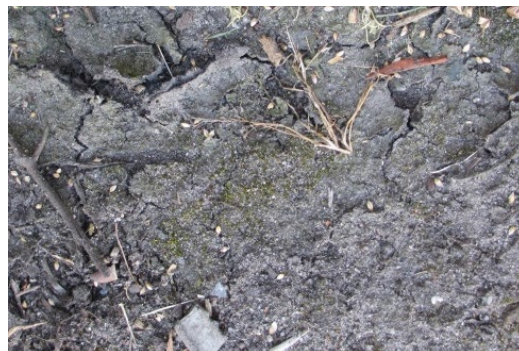
Clogging – build up of fine sediments, moss or plant litter on the surface reduces infiltration and treatment
