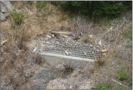
Blocked overflow grate – can lead to flooding and damage to the filter and vegetation
