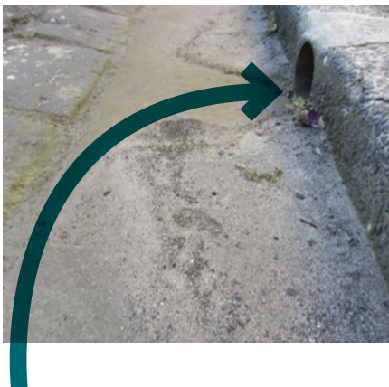
Sediment management: high risk of sediment washing into biofilter during construction in catchment
