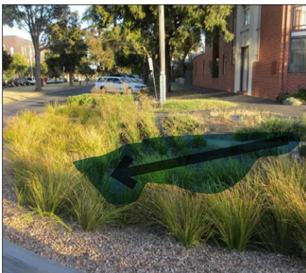
Batter slopes serve a purpose for safety, but need to be factored into design – in this case, the outlet level relative to batter slopes allows only very minimal flow distribution
