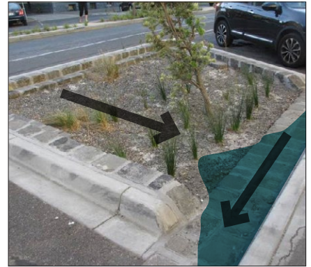
Slope follows road Biofilter surface not flat – uneven flow distribution and poor channelling of flows to top of system
