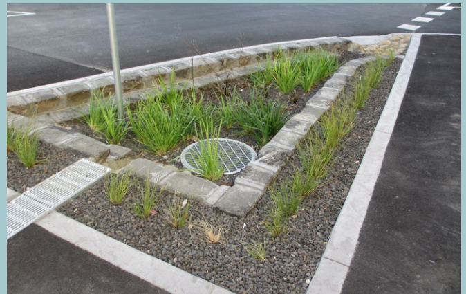
A stepped design, edge planting or batter slopes help protect pedestrians from the drop down into the biofilter for systems alongside pathways
