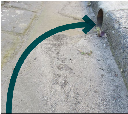
Sediment management – high risk of sediment washing into biofilter during construction activities
