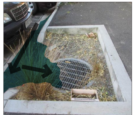
Outlet too close to inlet Outlet level too low – no ponding
