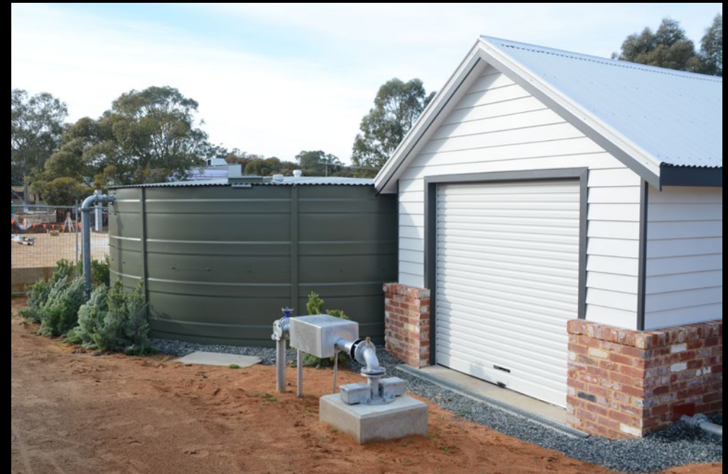
↑ Community groundwater bore pump house and storage tank (February 2017).
