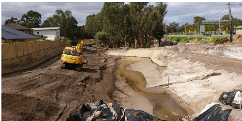
Channel reconstruction, Brentwood Living Stream, Western Australia. Photo: Glen Byleveld. Courtesy of SERCUL and WA Department of Biodiversity and Conservation
