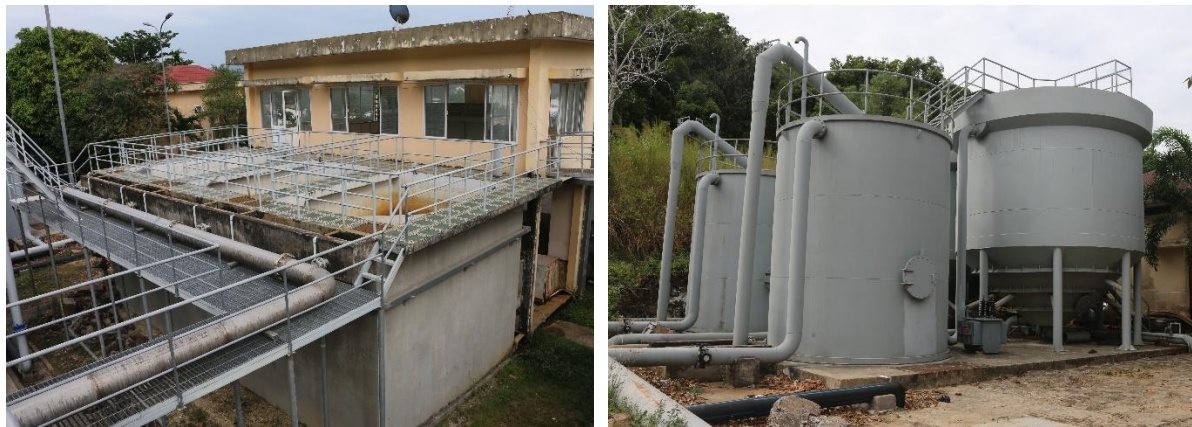
Figure 5: Existing Duong Dong WSS.
