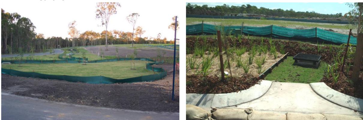
Figure 2. Protection of filter media with a geofabric and turf cover (left) and use of a sacrificial sediment forebay during construction and plant establishment (right).
