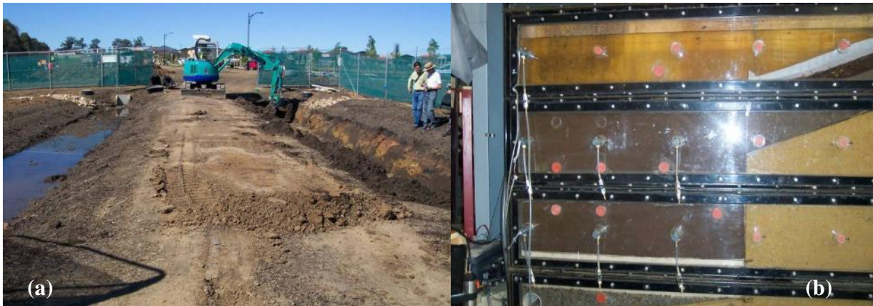
Figure 7. Second Ponds Creek bioretention system: (a) construction of the two bioretention trenches and (b) laboratory study of the performance of bioretention systems built in sodic soils
